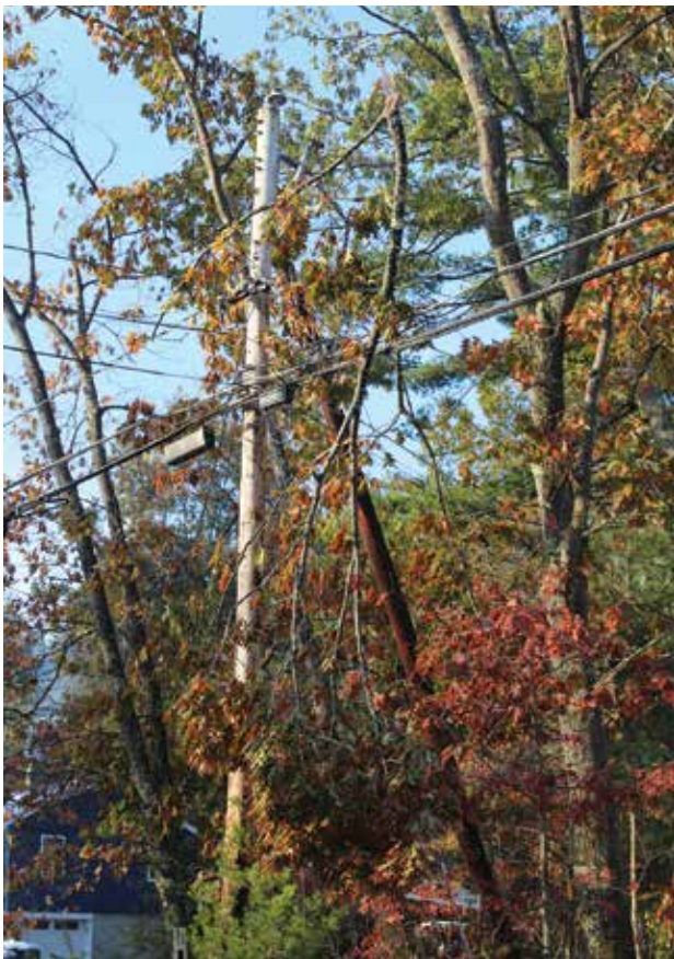
Example of an electrical hazard.
