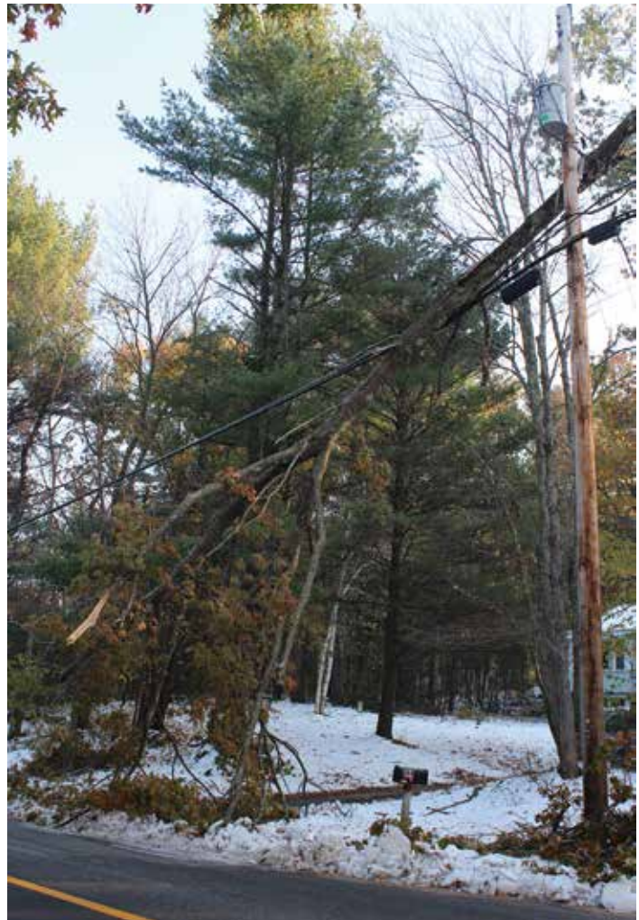
Phase-to-ground faults can be created by a tree touching a primary. Touching an energized tree could cause you to become part of the circuit.
